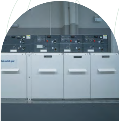
Backup power generators to guarantee business continuity.
